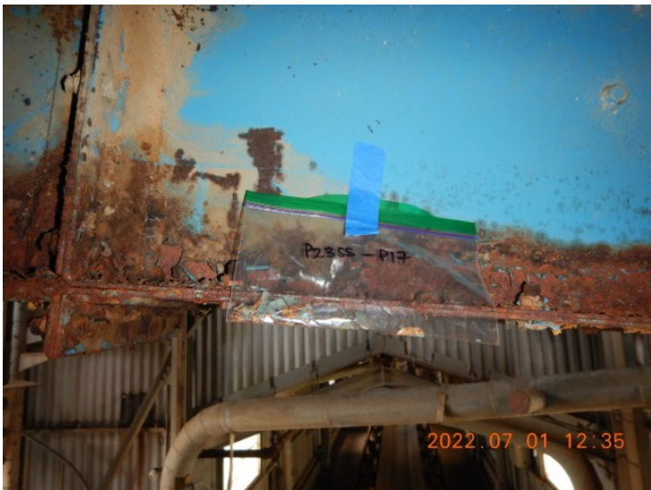
Photo 129 - P23SS-P17 (Close-up) [AL\DSCN6983.JPG]
