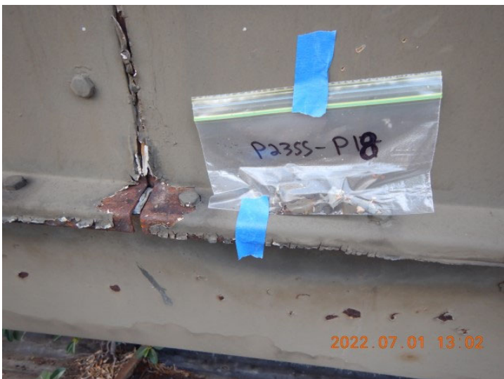
Photo 131 - P23SS-P18 (Close-up) [AL\DSCN7021.JPG]
