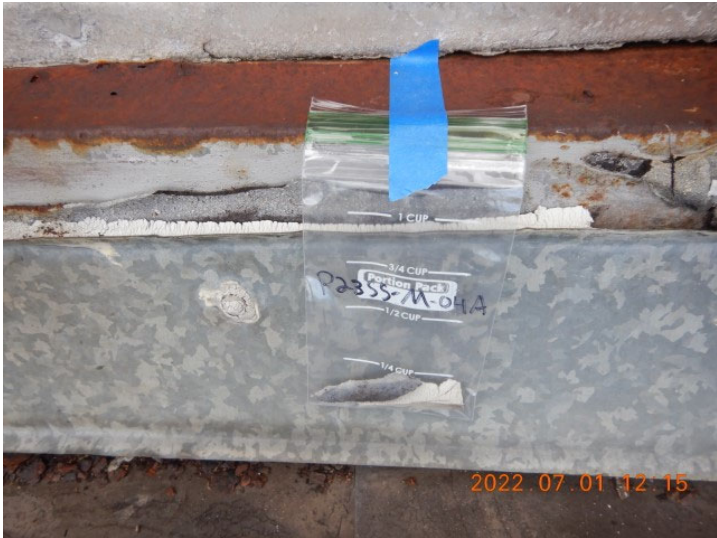
Photo 51 - P23SS-M-04A (Close-up) [AL\DSCN6966.JPG]
