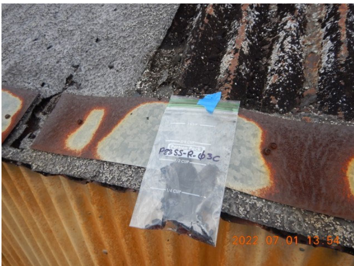
Photo 95 - P23SS-R-03C (Close-up) [AL\DSCN7061.JPG]
