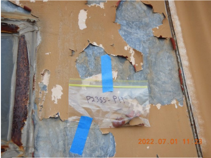
Photo 117 - P23SS-P11 (Close-up) [AL\DSCN6926.JPG]
