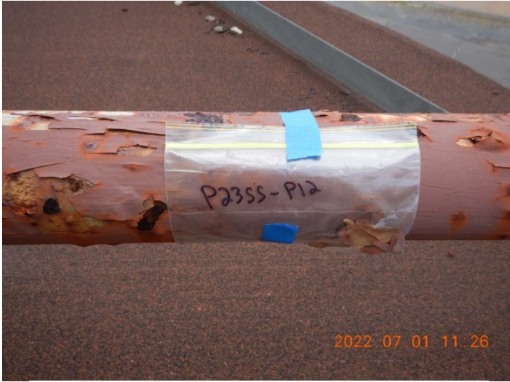
Photo 119 - P23SS-P12 (Close-up) [AL\DSCN6928.JPG]
