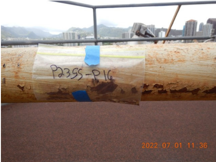
Photo 127 - P23SS-P16 (Close-up) [AL\DSCN6935.JPG]
