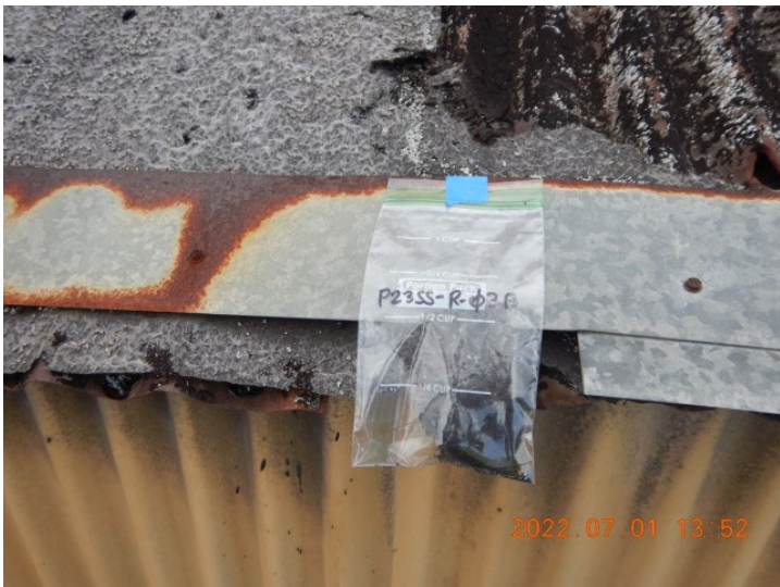
Photo 93 - P23SS-R-03B (Close-up) [AL\DSCN7059.JPG]
