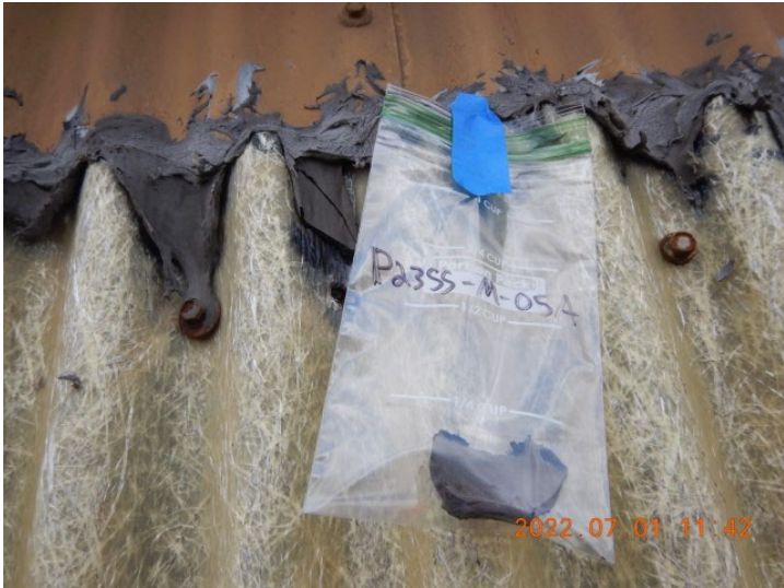
Photo 57 - P23SS-M-05A (Close-up) [AL\DSCN6942.JPG]
