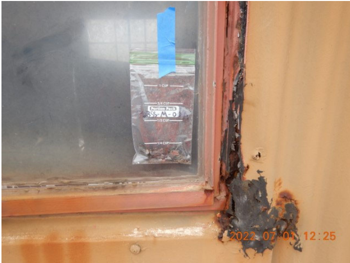
Photo 63 - P23SS-M-06A (Close-up) [AL\DSCN6976.JPG]
